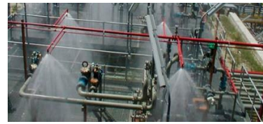
Gambar 4. Sistem Deluge Sprinkler
